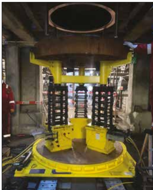
◀ Heat exchanger maintenance job on the piping and condensers at a refinery using a combination of Enerpac Heavy Lifting Technology: SCJ-Series Cube Jacks, the ETT-Series Hydraulic Turntable and LH-Series Low-Height Skidding Systems.
